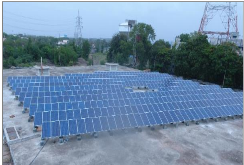
Photograph 1: 145kWp Solar PV System in Aji Water Treatment Plant
