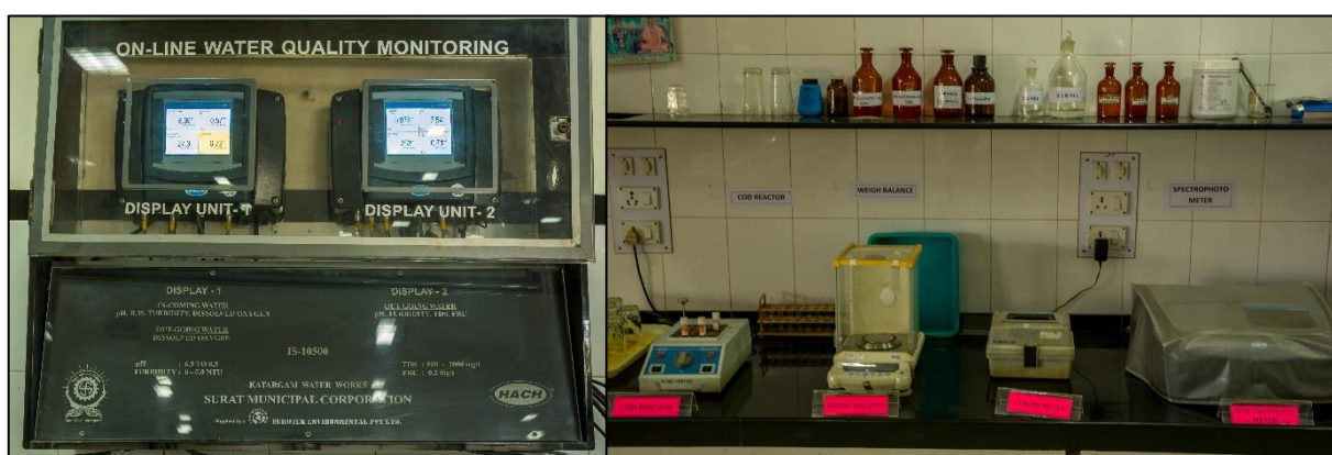
Figure 4-1: Online monitoring and analyzing equipment at Katargam
