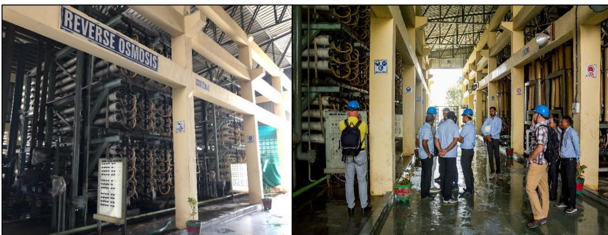
Figure 3-5: Reverse osmosis and ultrafiltration in Bamroli tertiary treatment plant
