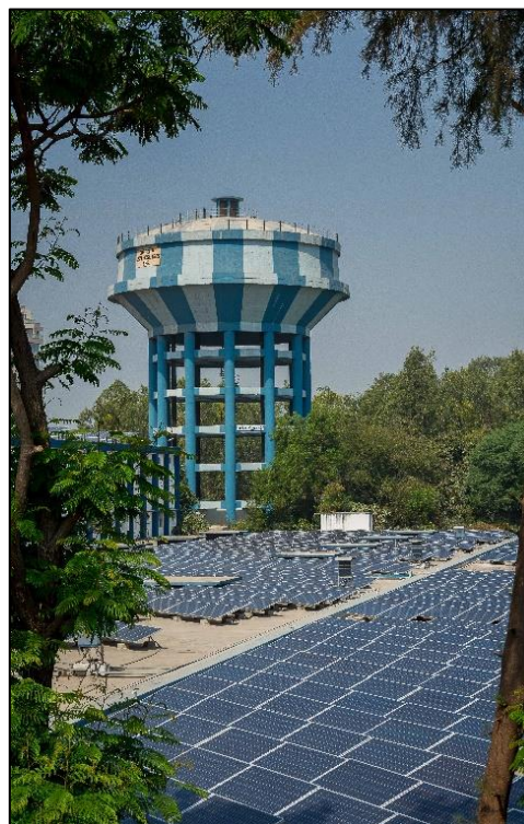
Figure 8-5: Solar panels at Katargam water treatment site
