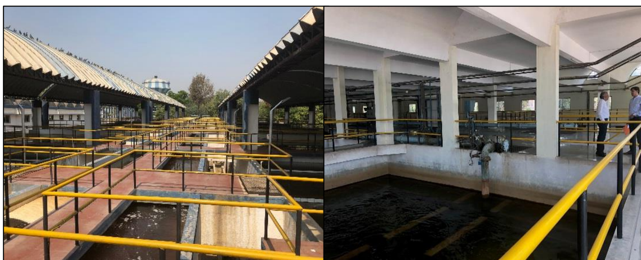
Figure 3-2: Clarification and filtration at Katargam treatment plant
