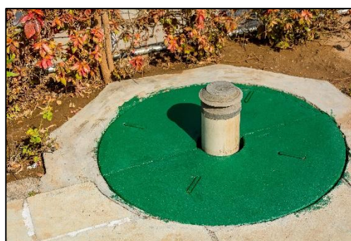
Figure 2-4: Rain water harvesting and infiltration system near Science Center
