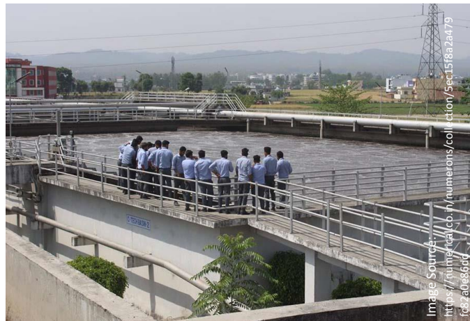
Photograph 1: Generation and treatment of sewage in Uttarakhand
